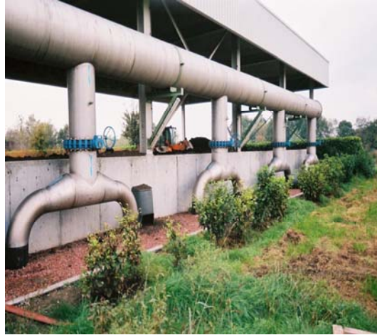
Back side of biofilter (Air cleaning system)
