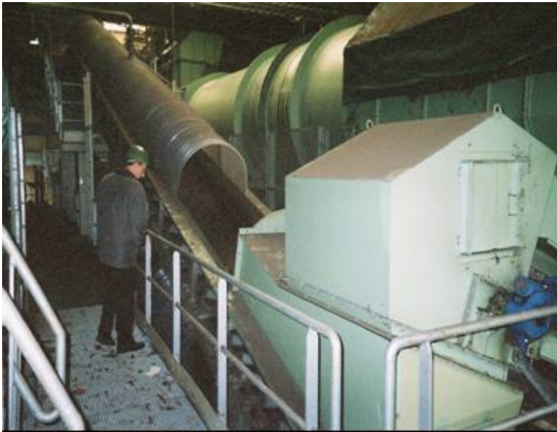
Comminuting drum in background, drum feed conveyor belt in foreground
