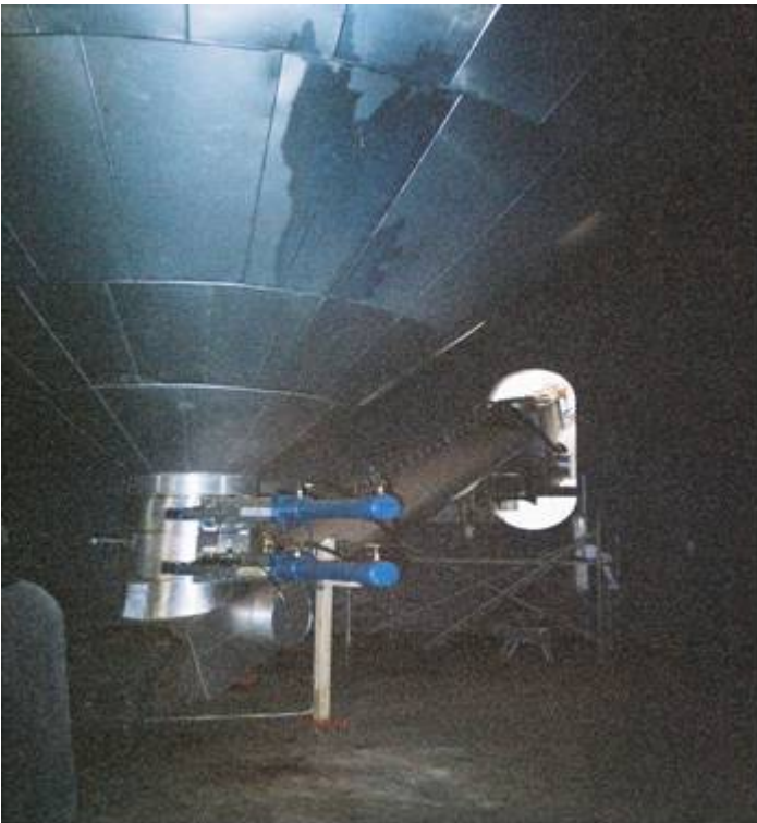
Conical digester bottom; the blue valves control the effluent rate; the pipe in background conveys effluent to the recirculation and mixing area
