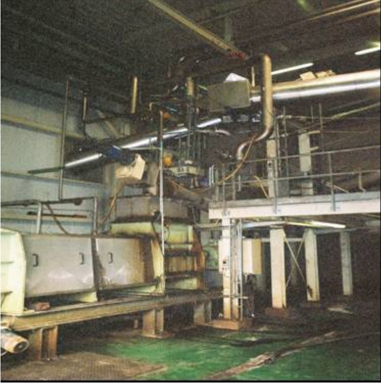
Digester effluent arrives in the recirculation and mixing area via the inclined pipe
