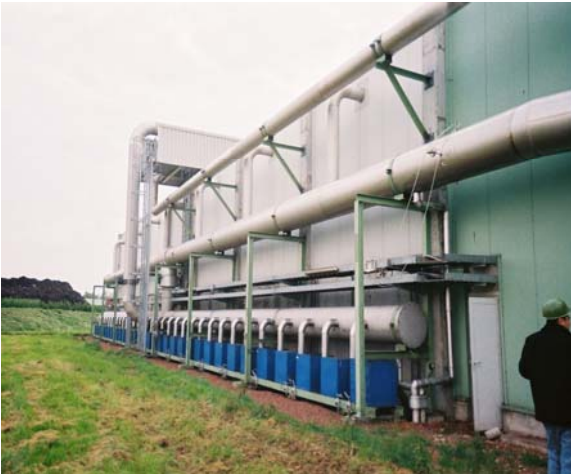
Air handling system, air from compost bays is injected into biofilter
